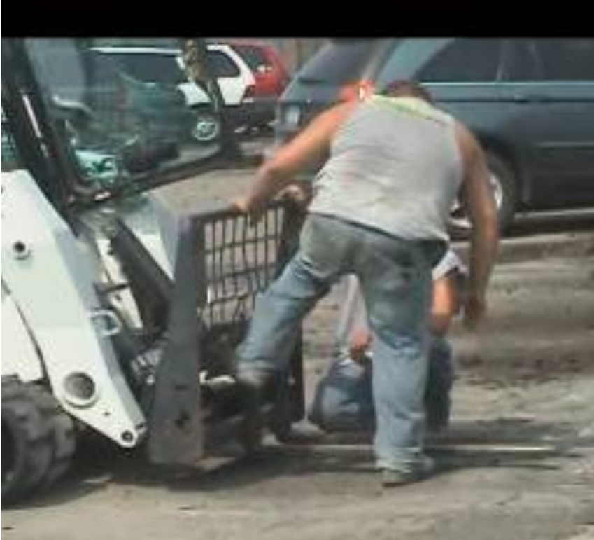
Figure 3 Unsafely kicking steel attachment, wearing tennis shoes
